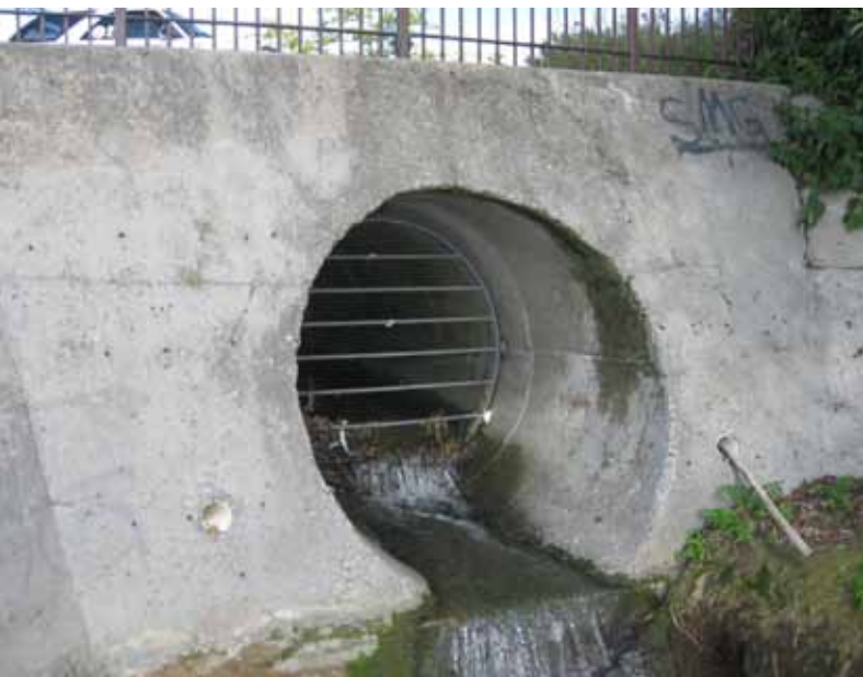
Combined Sewer Outfall
