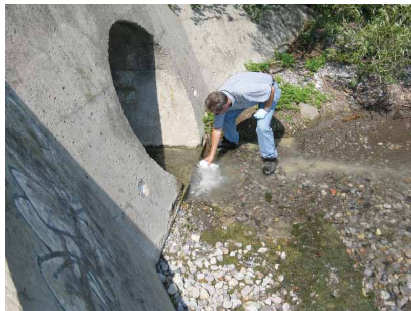
Water quality monitoring at an outfall
